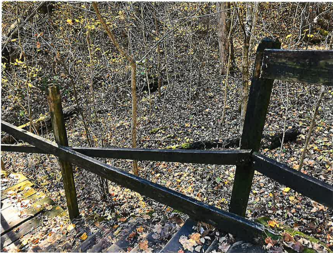
Broken railings on trails are not just unsightly, but also a safety issue.
